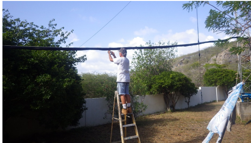
Each point gets two UV-resistant tie wraps, then the tie wraps must be covered by Scotch 33 tape. In Curacao, "UV resistant" means about six months. With the tape they will last indefinitely.
