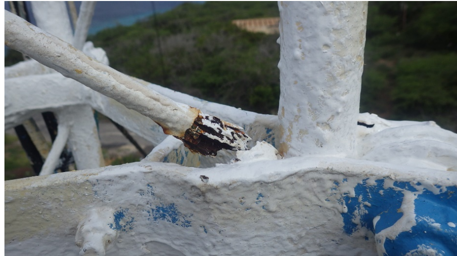
Broken zig-zag on the Europe tower.
