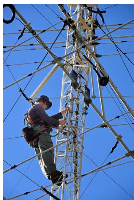
Jim W8WTS on the USA/JA tower, finding and replacing the blown-out PL-259 barrel on the 80-meter wire beam.
