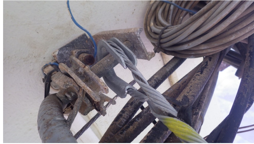
Photo shows the new deadend and thimble at the house. The clevis bolt goes all the way through the wall with a nut and washer above the radio closet.
