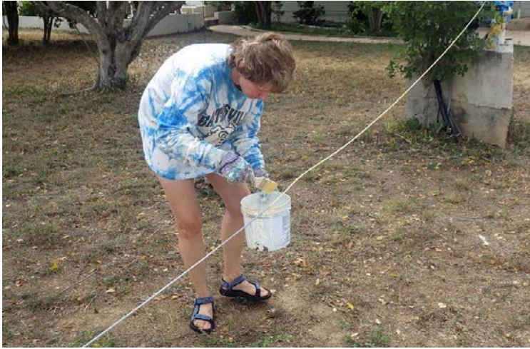
Dorothy and Geoff applied coats of epoxy paint to the new ¼-inch EHS messenger cable before stringing it from house to WARC tower.
